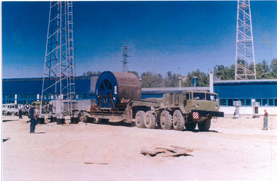
Pic. E1 Transportation of a cable drum fastened on a metal support structure
