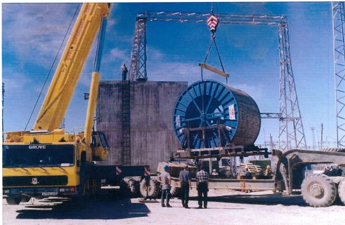
Pic. E2. Unloading of a cable drum fastened on a metal support structure
